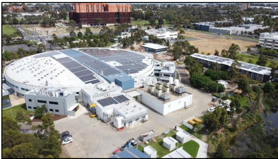
Figure 1: Australian Synchrotron site view showing the installation in progress of a 1.4 MW solar panel array, expected to generate up to 1.8 GWh/y. Photograph: Craig Millen (ANSTO).
